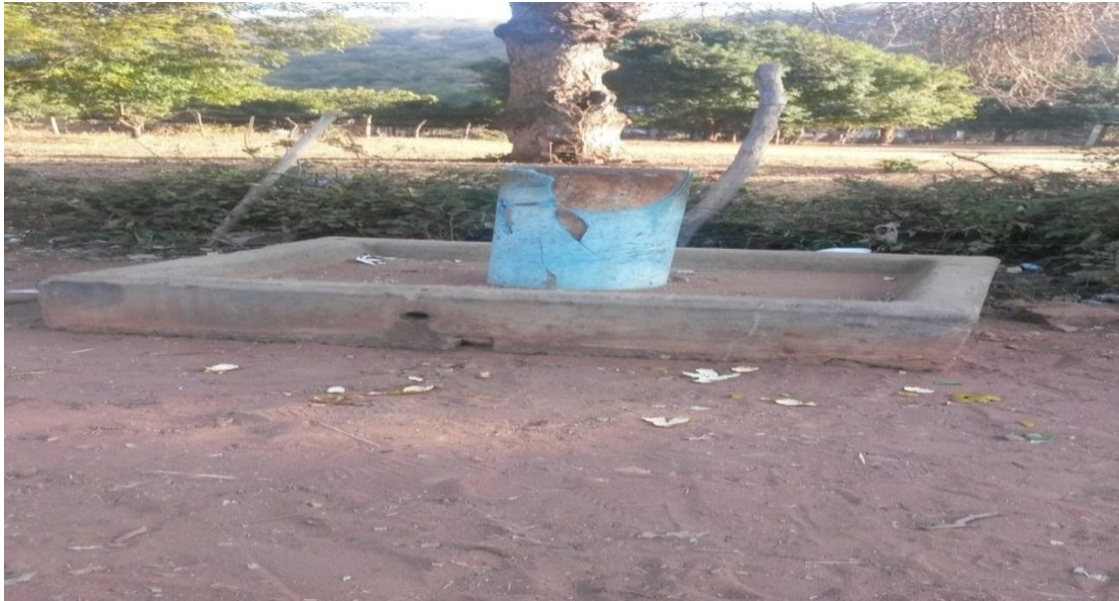
Picture 3. Poor pipelines maintenance in Mukondeni village
