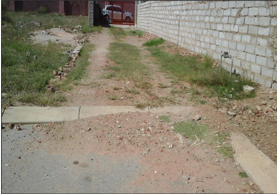
Figure 4.12: Lack of adequate access to connect the house and the street
