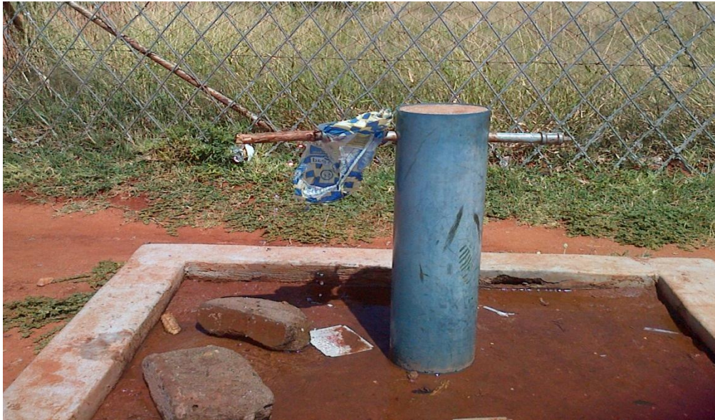
Figure 19: Leaking tap (b) in Mashite village
