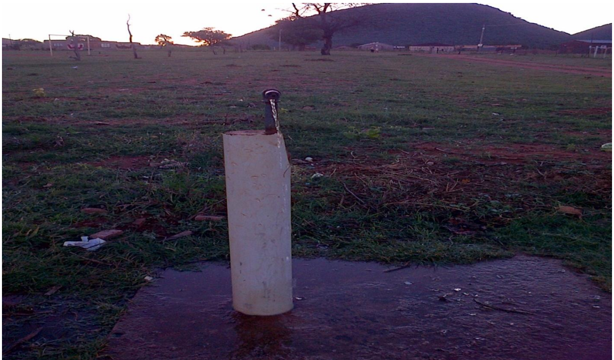
Figure 18: Leaking tap (a) in Mashite village
