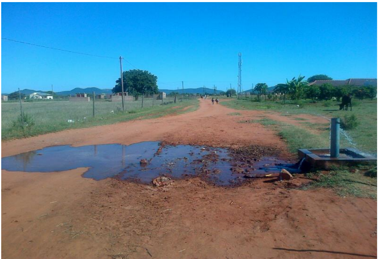
Figure 20: Leaking tap (c) in Mashite village causing damage to the road
