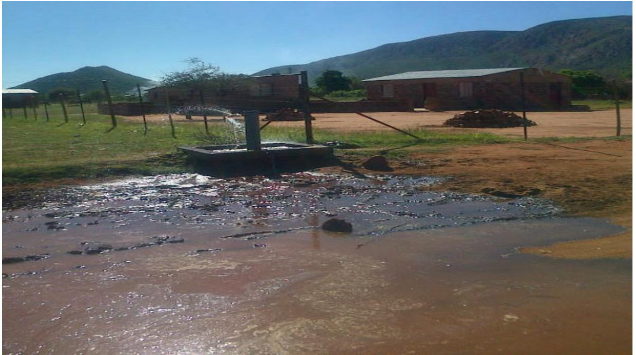
Figure 21: Leaking tap (d) in Mashite village causing damage to the roads
