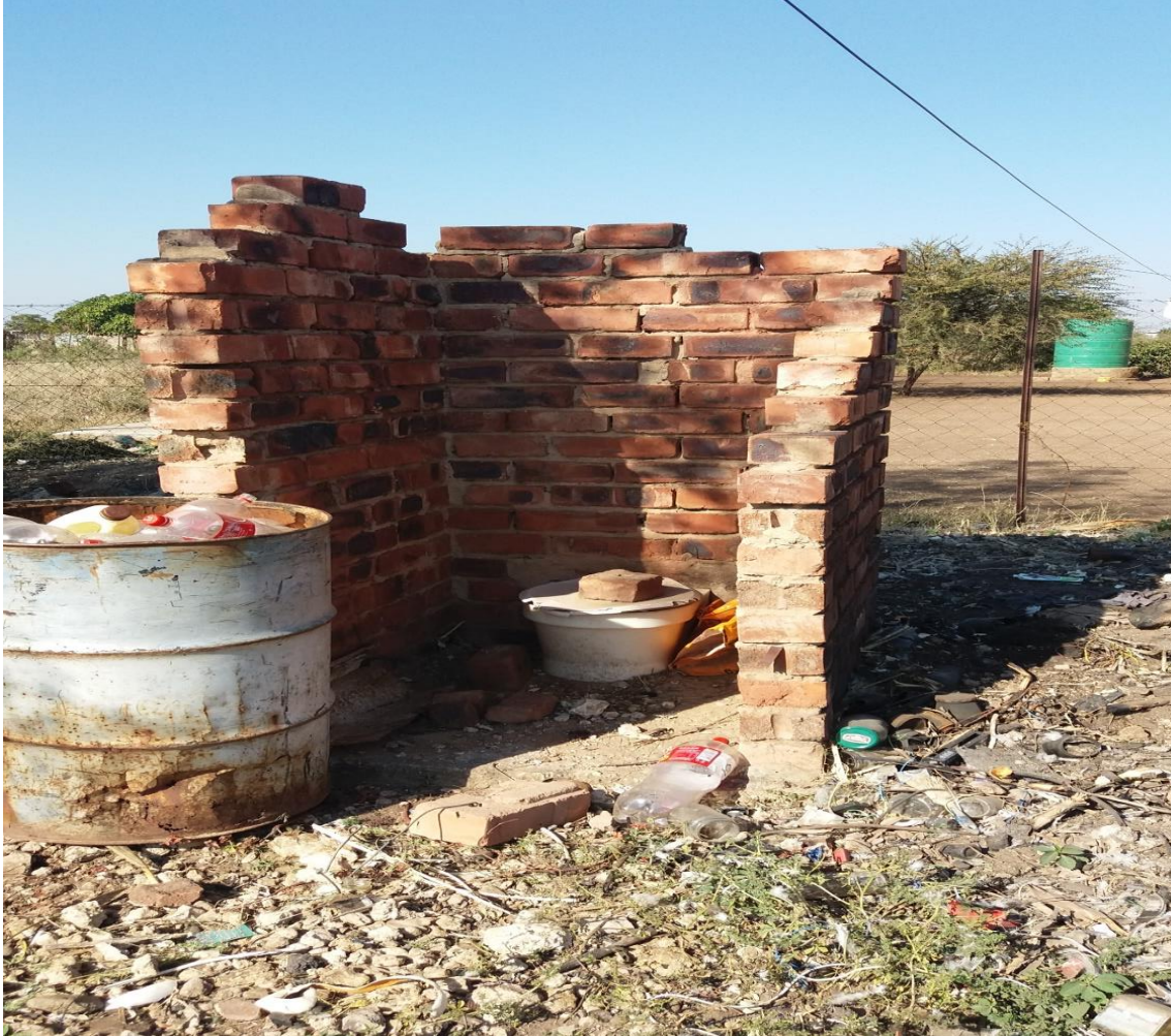
Figure 4.16: An illustration of dilapidated toilet
