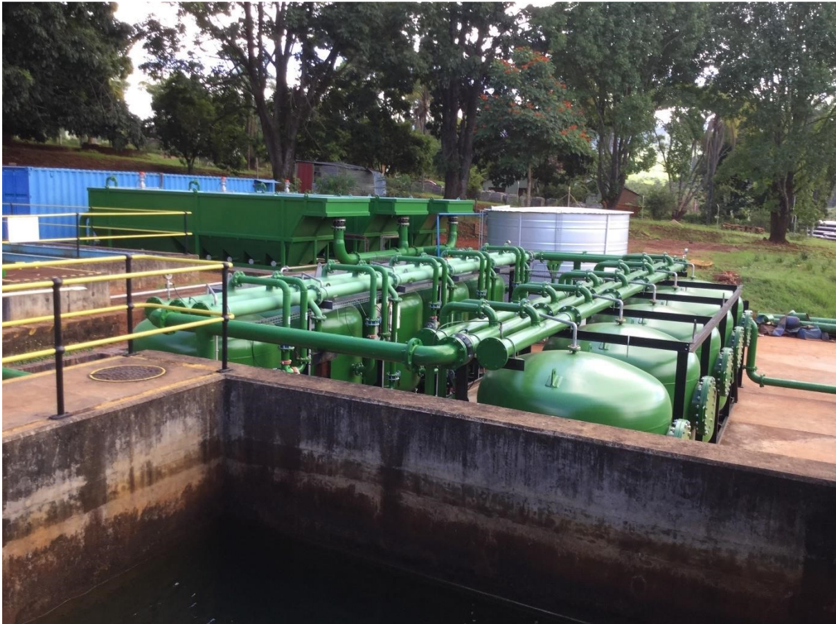
Figure 4.12: Showing picture of a New Politsi Water Purification package plant
