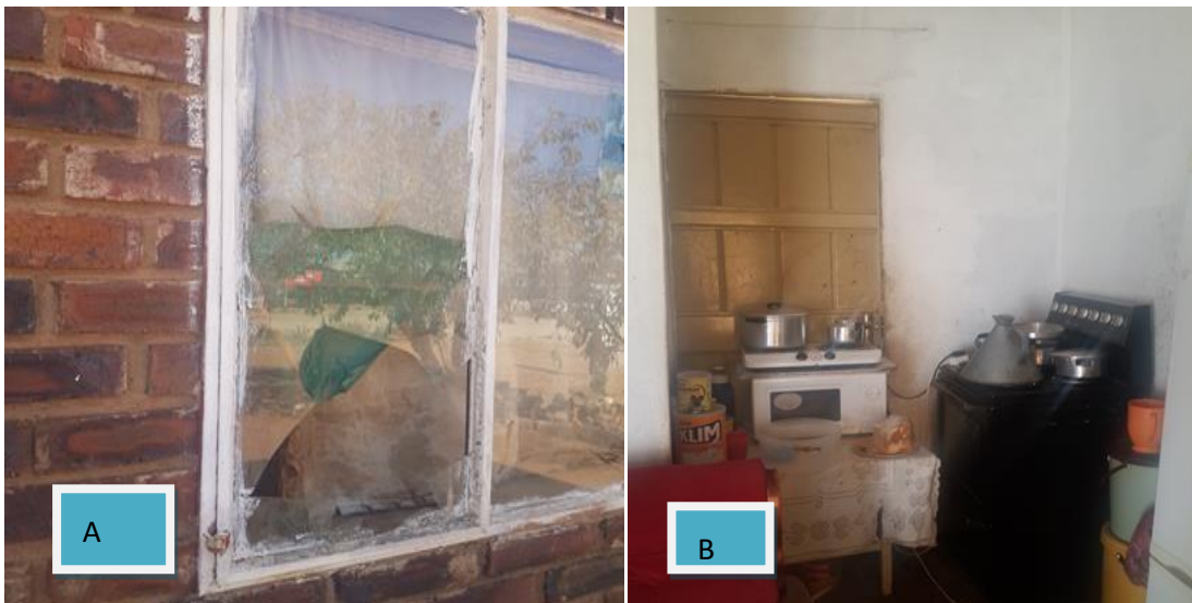
Figure 4.7 Depicting a broken window and small kitchen of an RDP house.
