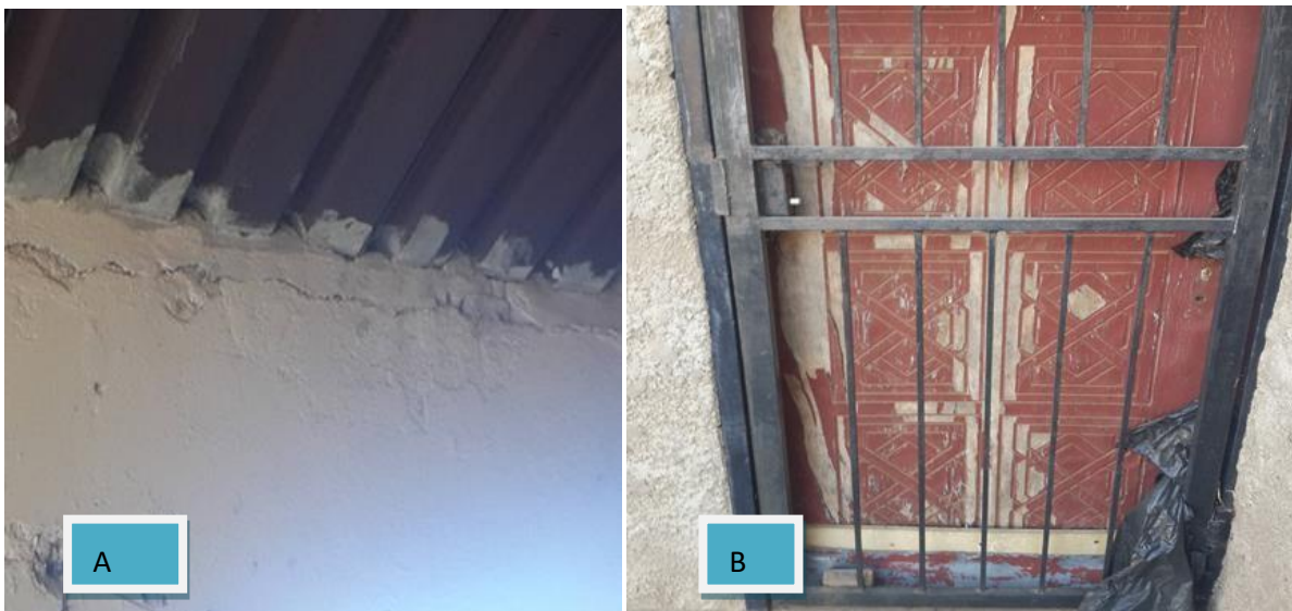
Figure 4.6 Cracked wall and doors covered with plastic
