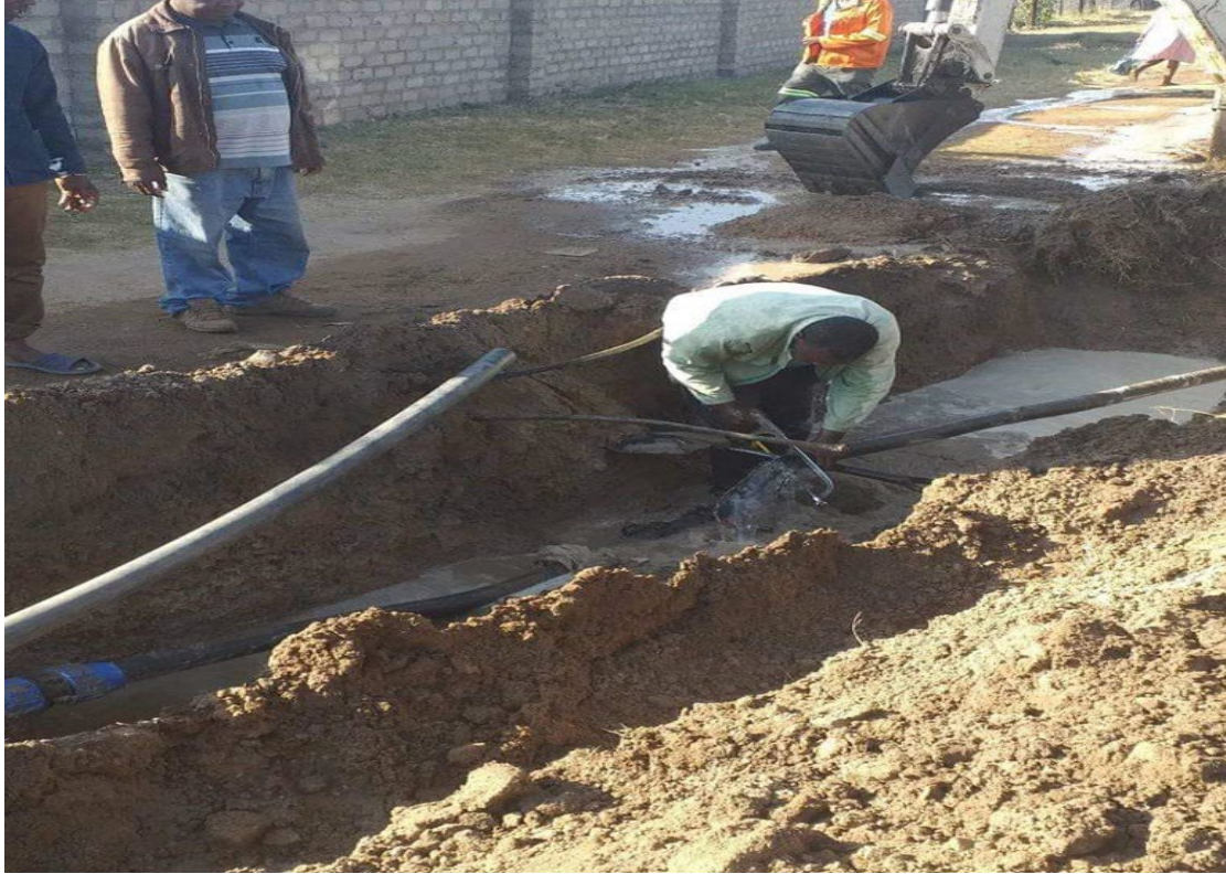
Figure 3: Community Members connecting water illegally from the main pipe
