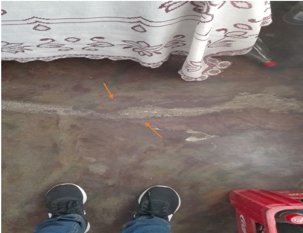
Figure 4.11: Cracked fixed floors from blasting and vibrations in Diphale village
