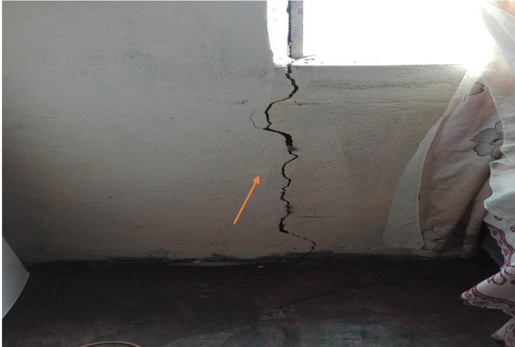
Figure 4.12: Cracked wall from blasting and vibrations in Diphale village
