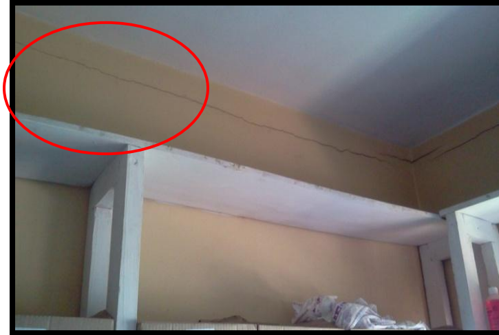
Figure 4.5: Cracks in medicine store wall at a clinic (Clinic C).
