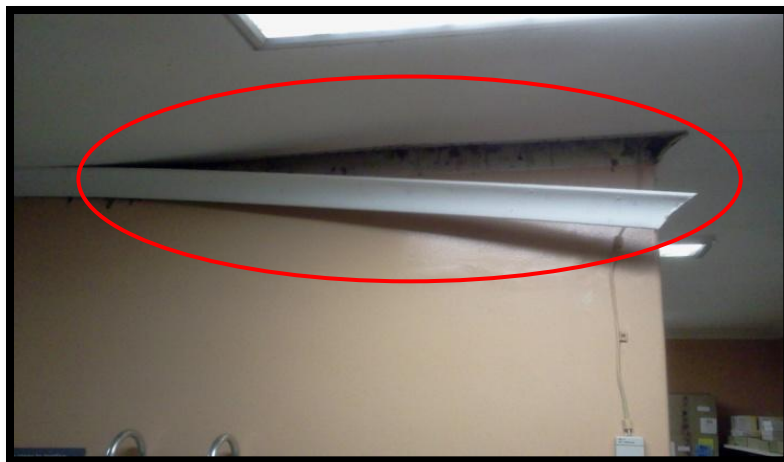
Figure 4.6: Broken ceiling panel (Clinic D).
