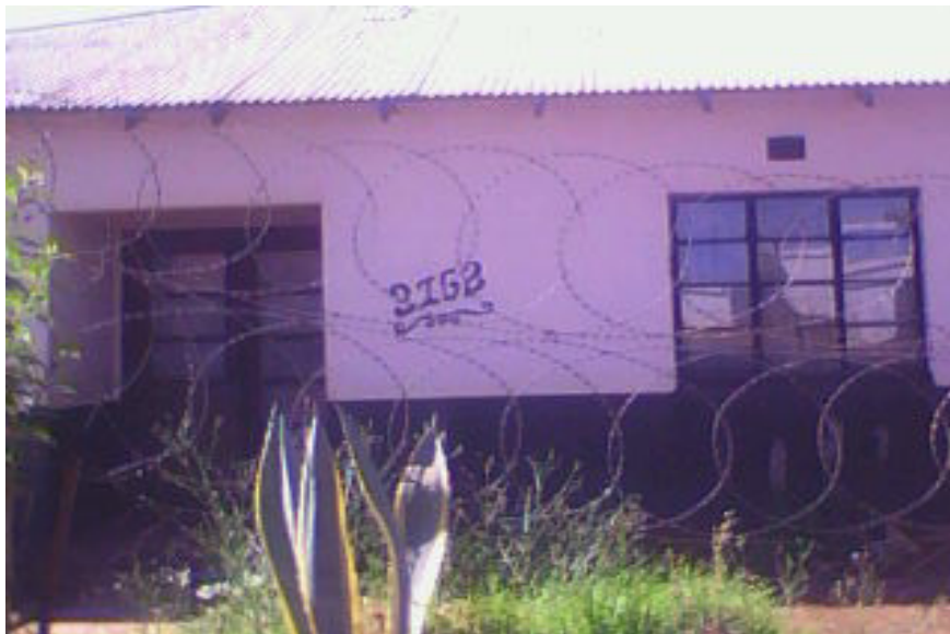
Photo 4.2 Old house with corrugated iron roof upgraded to the standard of the new houses in Protea South
